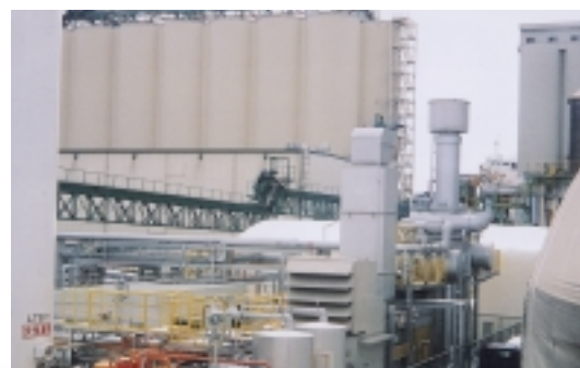
Co-generation Equipment (Kobe Plant)
